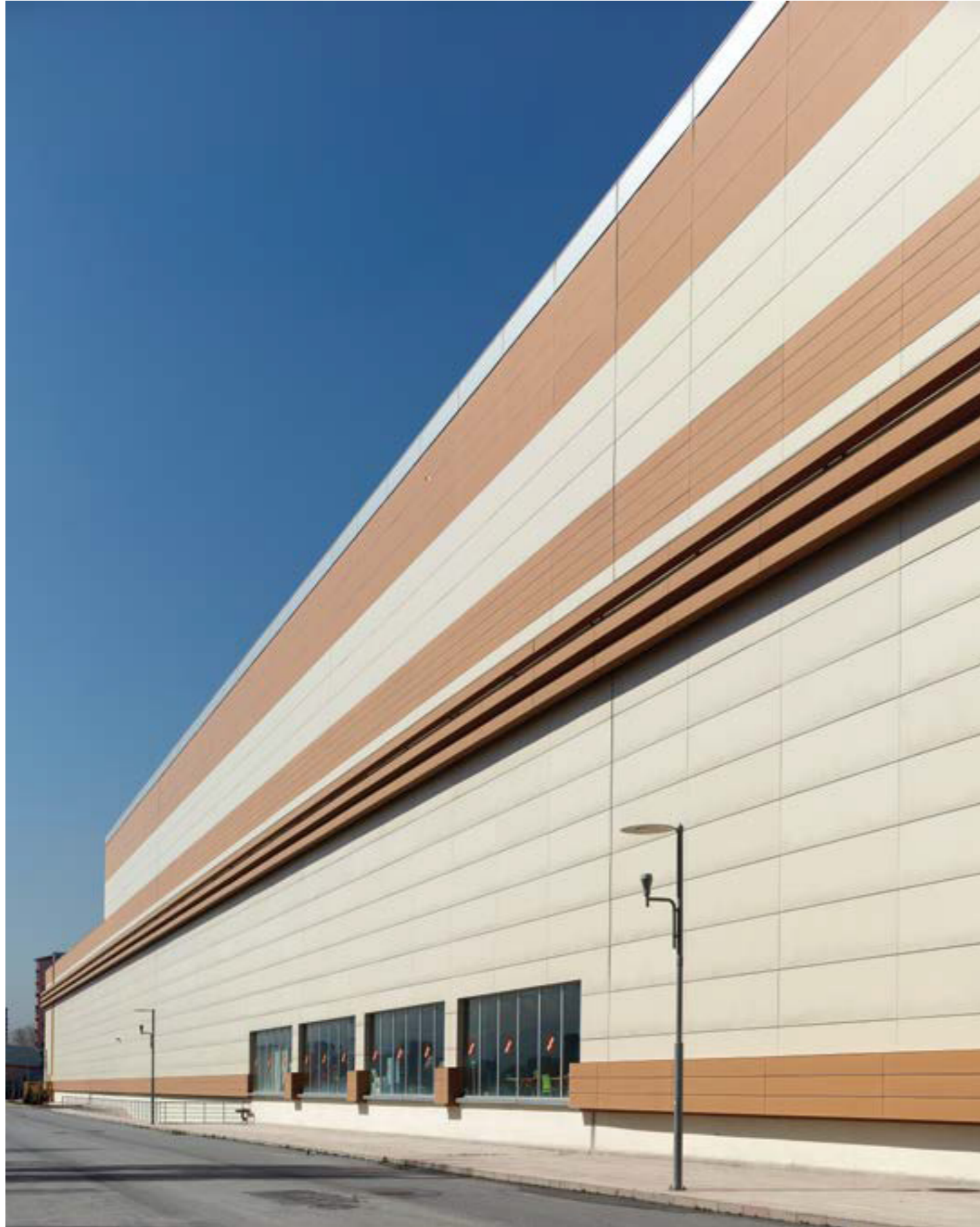
Kayseri Optimall AVM / Kayseri — 3mm Mat Fit Bej - 3mm Mat Fit Safran / Gizli Klipsli Sistem Kayseri Optimall Shopping Mall / Kayseri — 3mm Matte Fit Beige - 3mm Matte Fit Saffron / Hidden Clips Fitted Facade System
